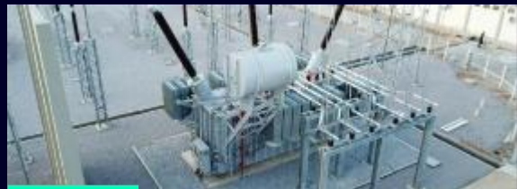
High Voltage Power transformers
