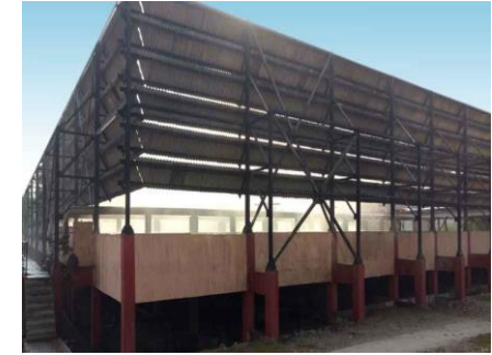
Mist Cooling System
