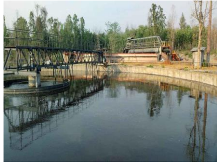
Secondary Clarifier - Pulp
