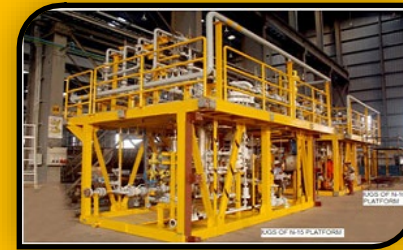
Instrument Utility Gas Drying Systems
