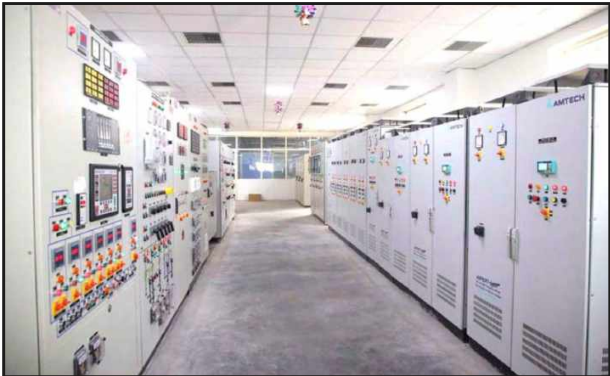
NEW MAIZE PROCESSING FACILITY COMMISSIONED IN PUNJAB
