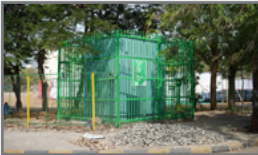
District Regulating Station
