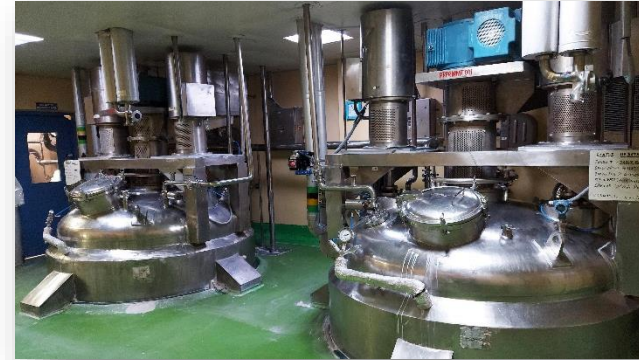
Main Mixing Tank
