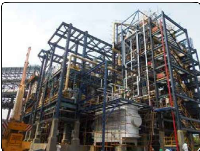
PA Plant Revamp : Oxidation Section - Ranipet
