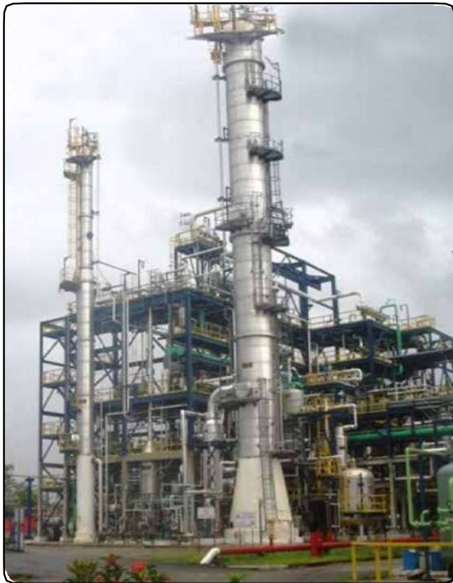
Butane Processing and Butamer Plant: Malaysia
