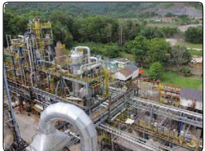
Maleic - Distillation Unit after Expansion : Malaysia
