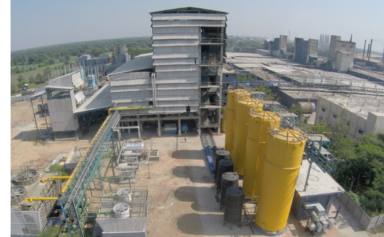
Multiple Effect Evaporator Plant (MEEP)
