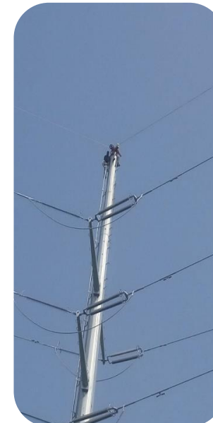
HTLS on pole
