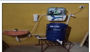
DRINKING WATER SYSTEM
