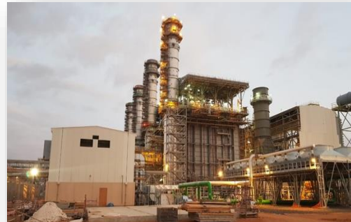
1,390 MW Waad Al Shamal ISCCPP, GE, KSA
