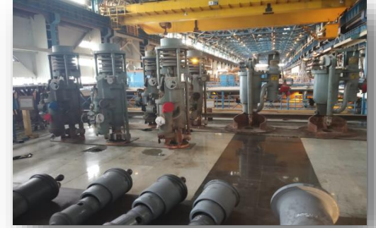
Control & Stop Valves Overhauling Sipat 660 MW
