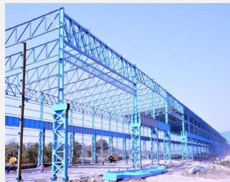
Viraj Steel Section Rolling Mill, Boisar
