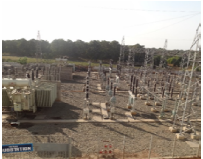
132KVA Sub Station
