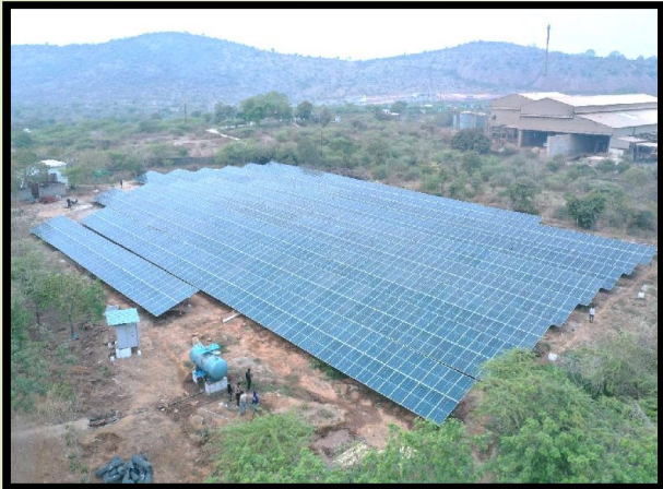
Solar Plant Udaipur
