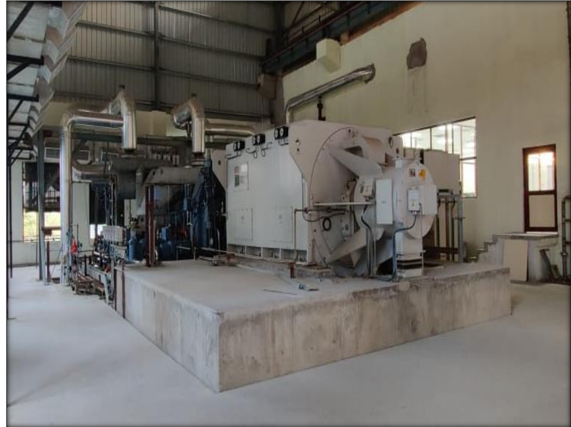
Steam Turbine Generator
