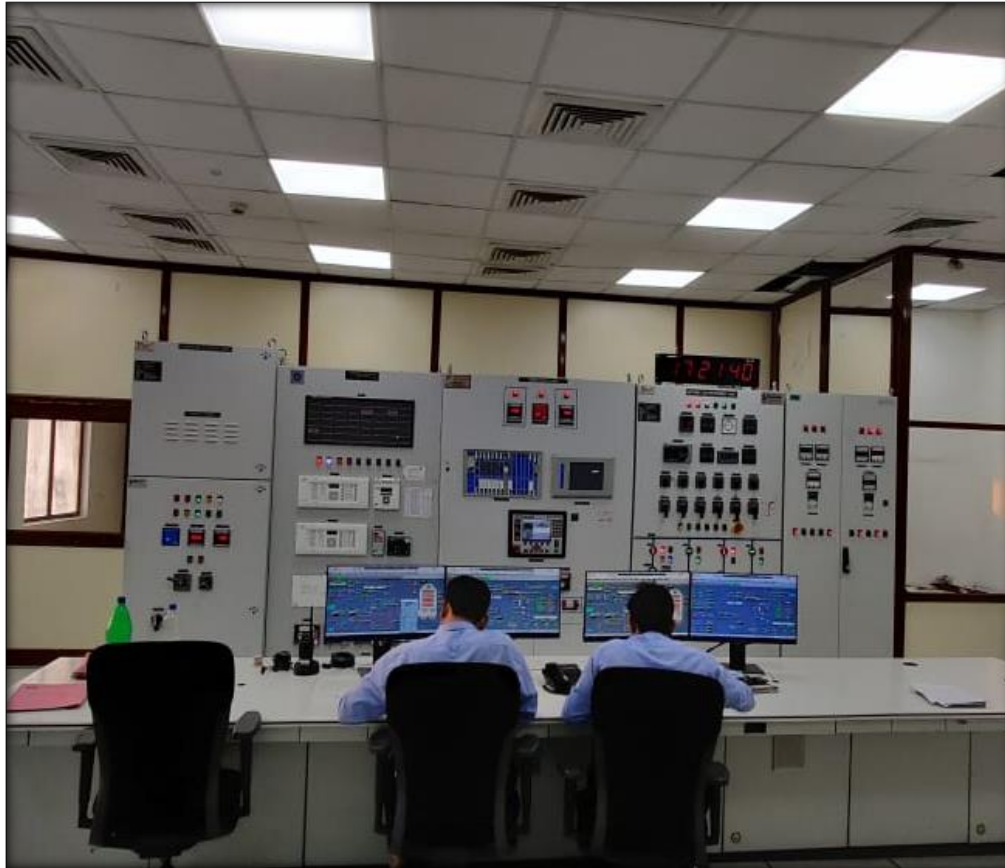
WHRS Control Room
