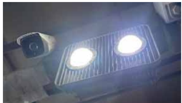
BRL's LED lighting system at Bharuch plant
