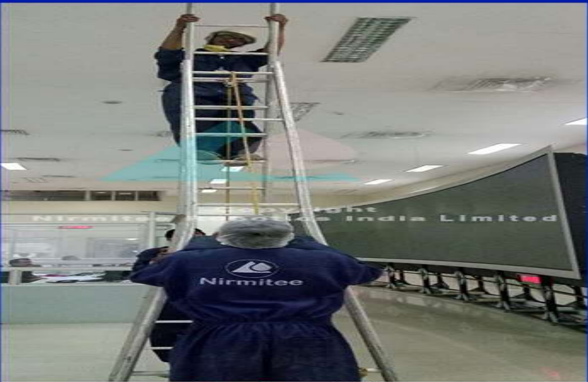
Our Speciality Critical Server and Projection Rooms
