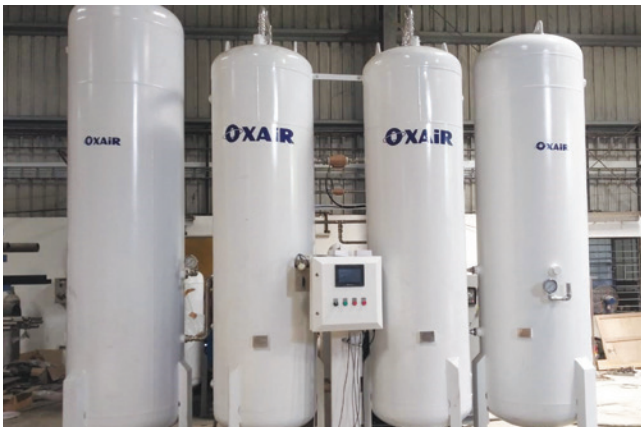
Oxygen generator plant
