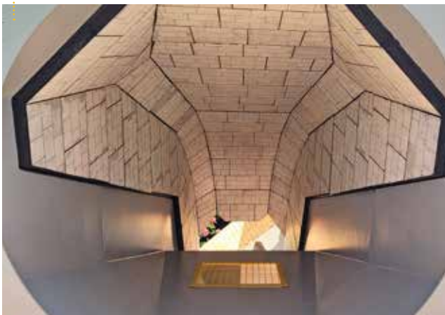
Internal view of ceramic lined surface of bauxite soft loading chutes
