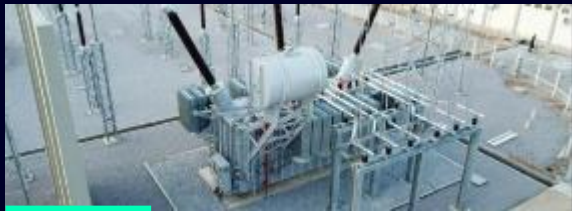
High Voltage Power transformers
