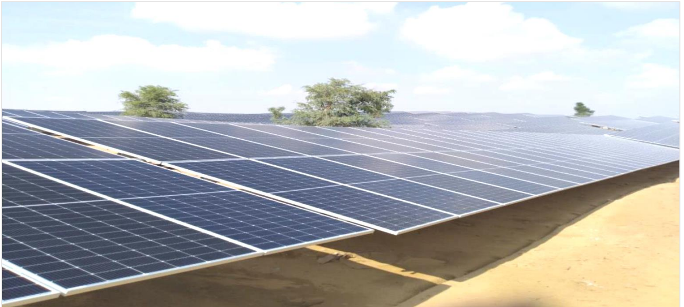
Image 1: 225 MW solar installation in Rajasthan
