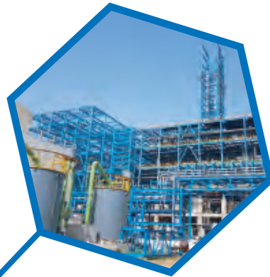
GACL Dahej Hydrazine Hydrate Plant
