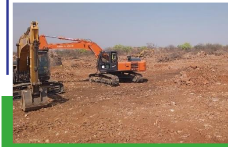
980 MWp at Kurnool, Andhra Pradesh
