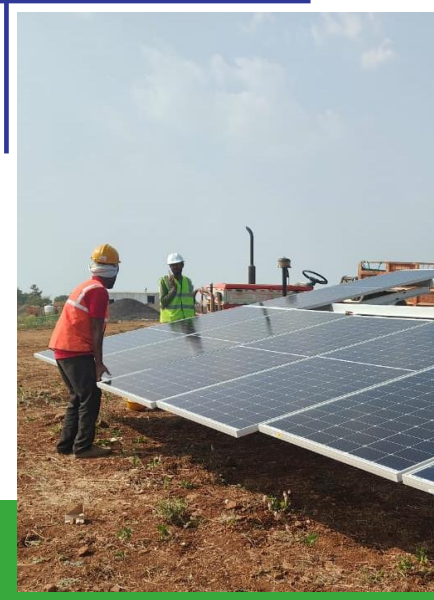
70MWp Ground Mounted project at Jalna
