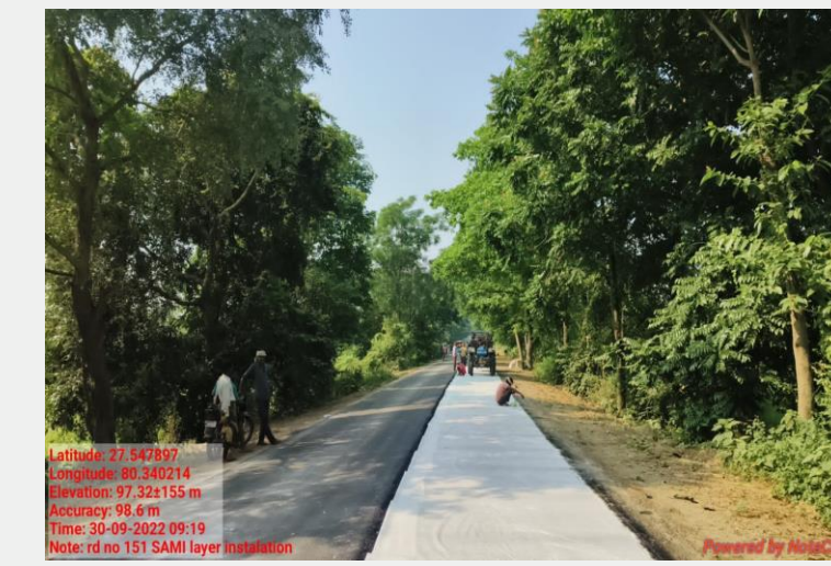
Laying of Paving fabric and Providing BC / PQC over the stabilized Layer
