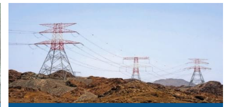
Transmission Lines, Fujirah, Dhaid
