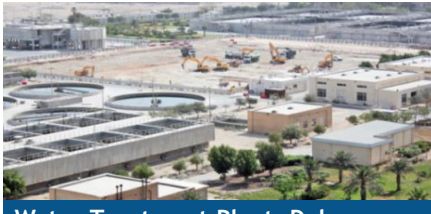
Water Treatment Plant, Doha
