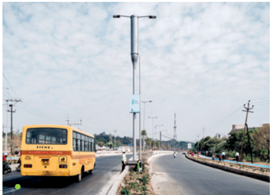
Multiple Smart Poles installed at a highway near Bhopal
