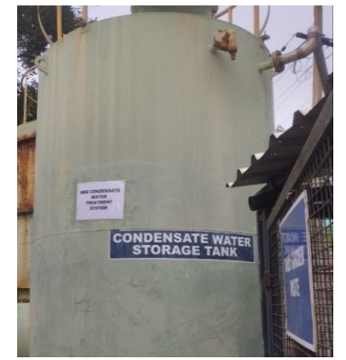
Condensated water recovery
