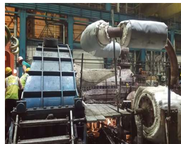
Emergency outage for vibration NTPC Sail #2- Durgapur plant
