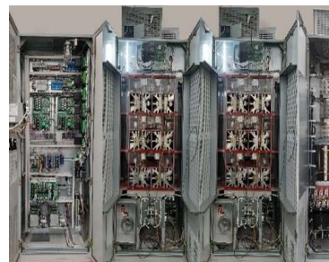
PAC excitation system completed FAT unit #1 Adani Godda 2x800MW
