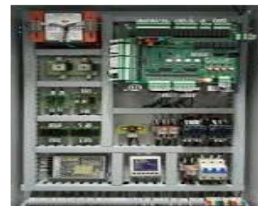
TG controller for UPRUVNL Obra completed FAT for unit 2, 2x660MW
