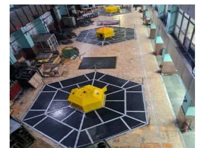
Bhabha 3x40MW hydro project synchronized to Grid
