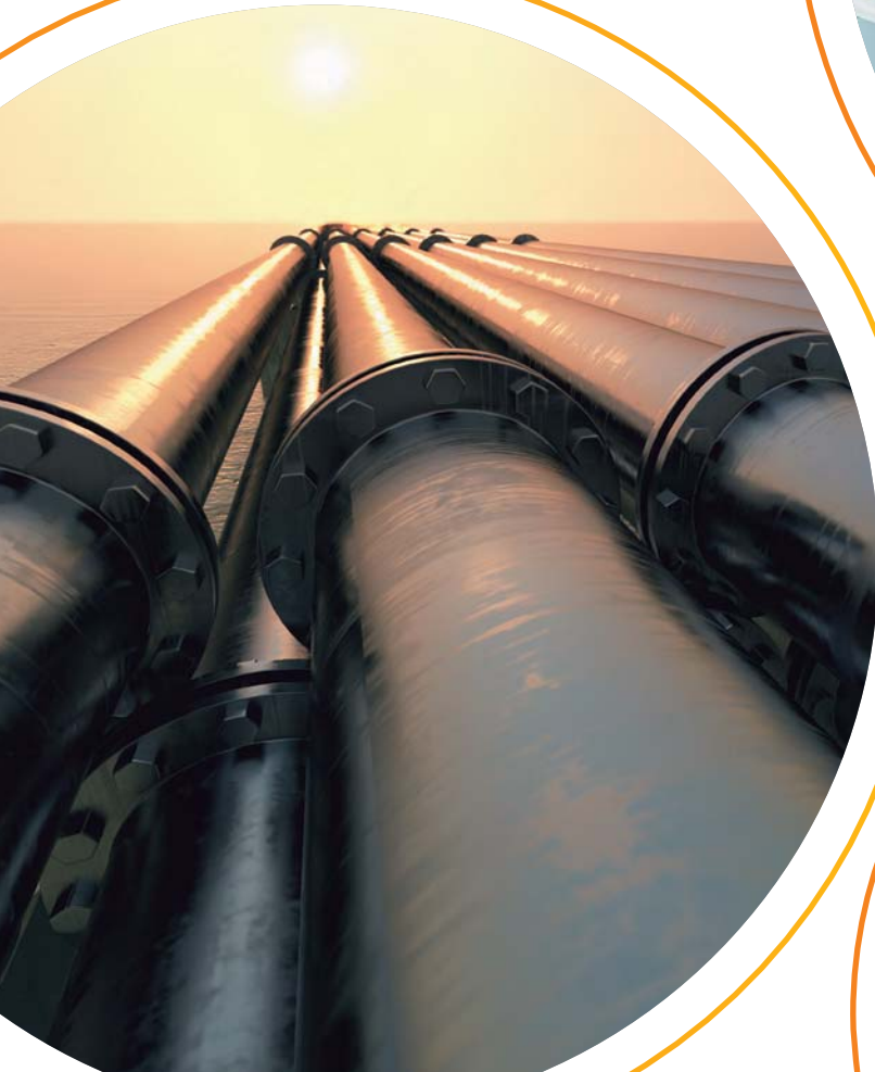
Oil pipeline infrastructure
