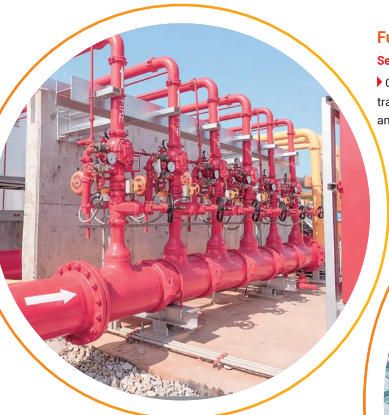
Fire fighting infrastructure
