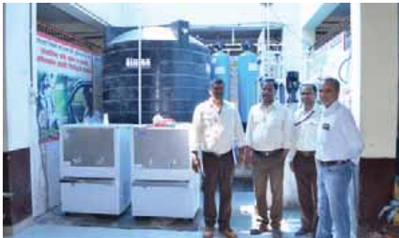
Water ATMs installed in Kanpur
