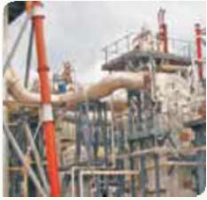
Tank Farm Heating
