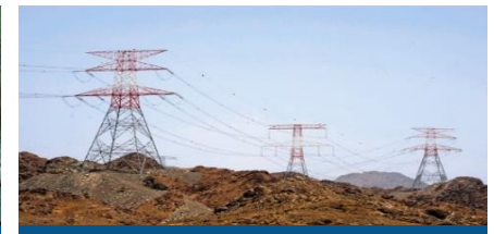
Transmission Lines, Fujirah, Dhaid
