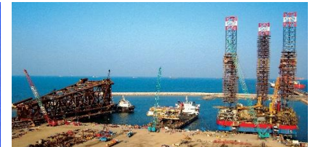
Fabrication Facility, Oman
