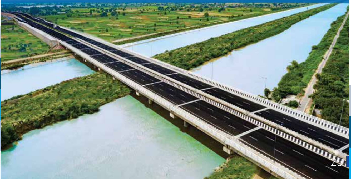
Construction of 6 Lane Canal bridge at Km 205.510 under Four Laning of Aligarh – Kanpur section package-II from Bhadwas – Kalyanpur of NH-91 in the State of Uttar Pradesh
