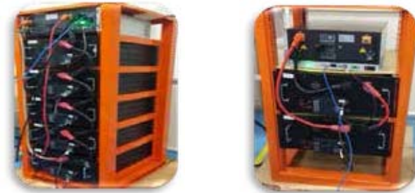
Energy Storage System (ESS)
