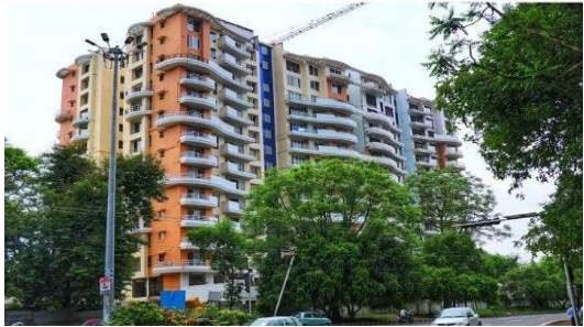
Construction of 96 flats at Tulsi Tower, Bhopal for MP Housing & Infrastructure Development Board
