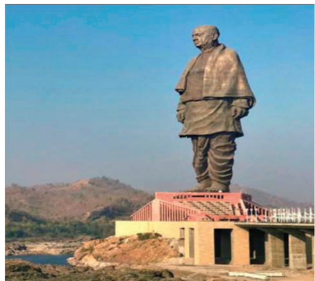
Protecting the world's tallest statue - KBL firefighting pumps have been installed at the "Statue of Unity"
