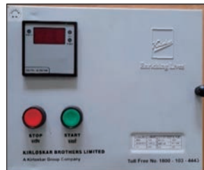
Microcontroller based panels for submersible pumps
