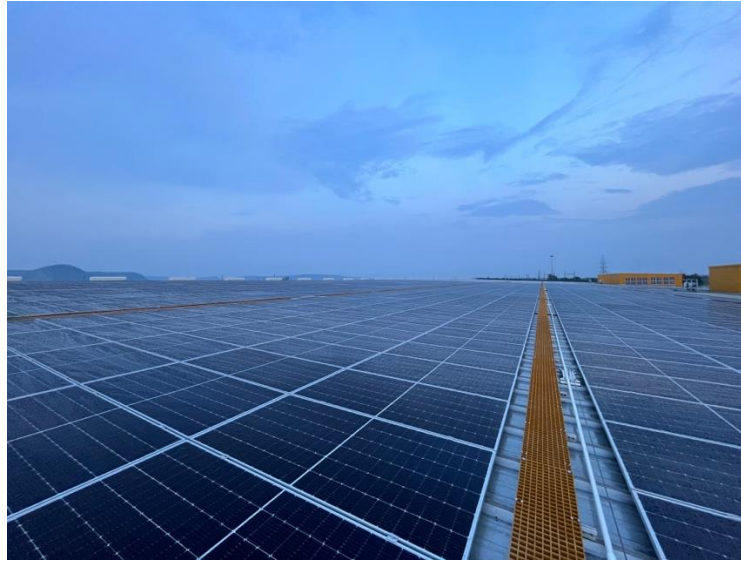
Photo caption: 10.6 MWp single Rooftop Solar project at Trident's Budhni plant, Madhya Pradesh.
