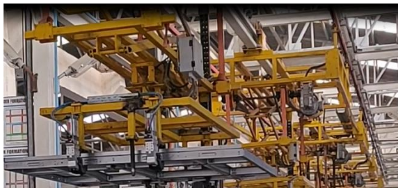
Material Handling System for Line Mode
