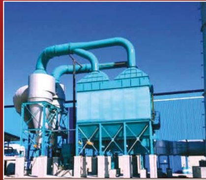
Air Pollution Control Equipment
