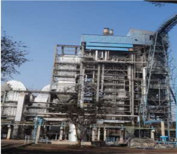
60 MW Captive Power Plant
