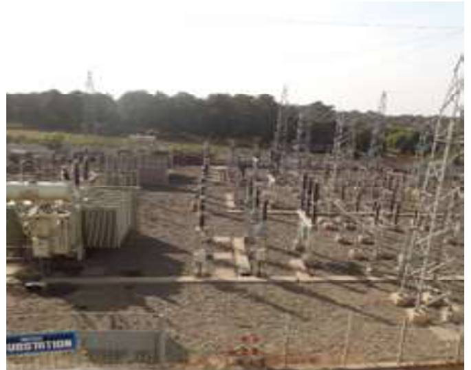
132KVA Sub Station
