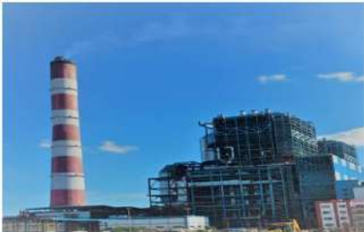
2x500 MW Neyveli TPP, NLC
