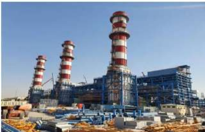
Aweer Power Station H Phase IV, Elsewedy, Dubai
