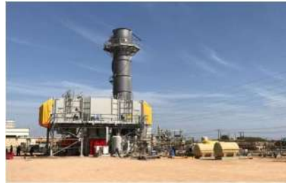
25 MW, Ray Project-RAY International LLC, Oman
