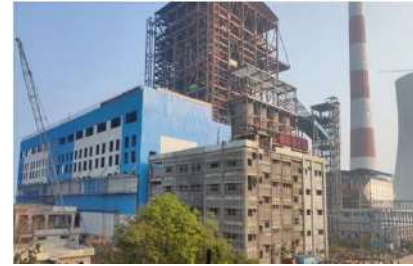
1x800 Mw TPSS, North Chennai, TANGEDCO
