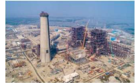
2X660 MW at Rampal, Maitree, Bangladesh-BIFPCL
