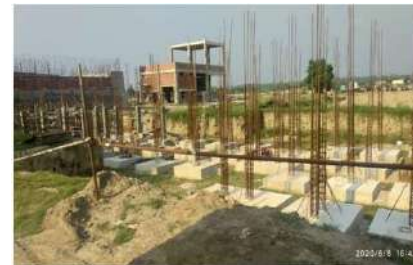
28 MLD STP at Karnal, TPL
