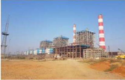
3x660 MW Nabinagar STPP, NPGCL
