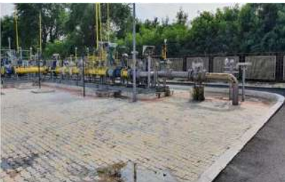
Station Piping at Ennore, IOCL
