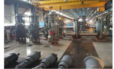
Control & Stop Valves Overhauling Sipat 660 MW
