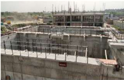
27.5 MLD STP, Networking at Palwal, MCPALWAL
