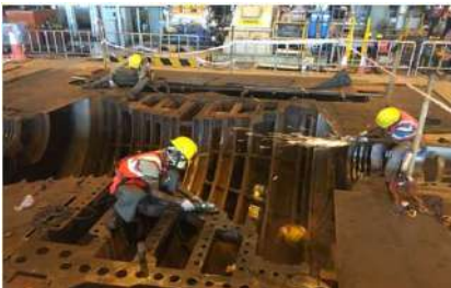
Main Turbine Overhauling, 660 MW, Kawai
