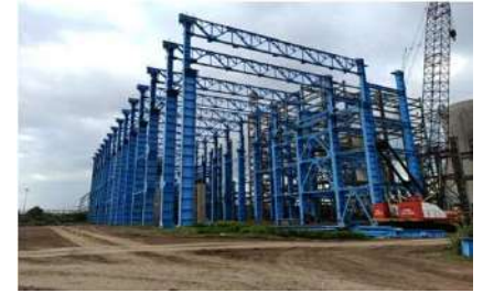
1X660 MW Bhusawal TPS at Maharastra-MAHAGENCO
