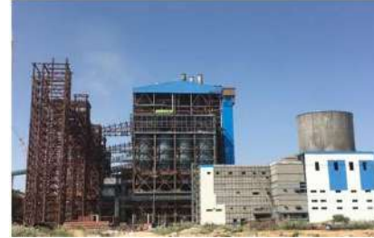
2x660 MW Suratgarh STPP, RRVUNL
