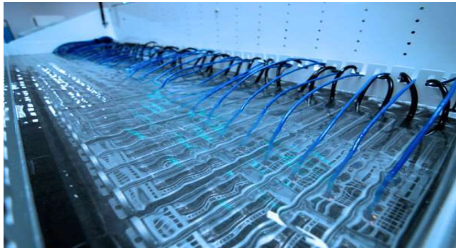
DATA Centre Cooling
