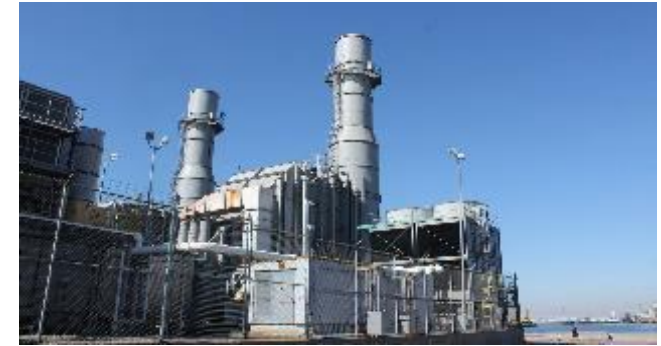
Captive Thermal + Waste Heat Plants (Total capacity of 161.5 MW)
