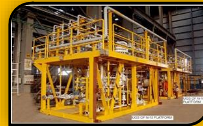
Instrument Utility Gas Drying Systems
