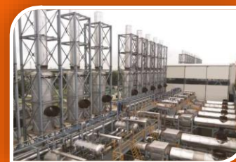
200 MW Combined Cycle power Plant
