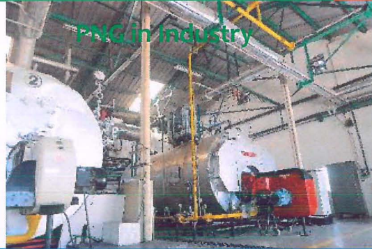
Natural Gas Skid
