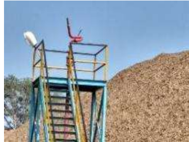
Fire Hydrant Point near chipper
