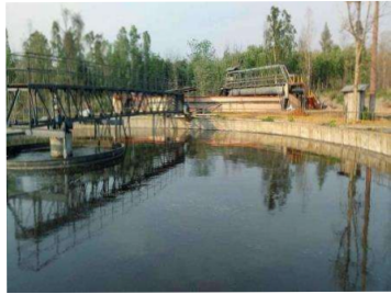
Secondary Clarifier - Pulp
