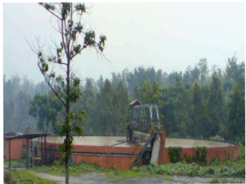
Primary Clarifier - Pulp
