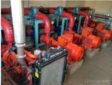
Fire Hydrant Pumps
