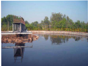
Primary Clarifier - Paper
