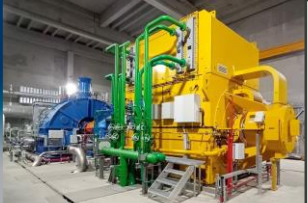
Steam Turbine Generator & Site Installation
