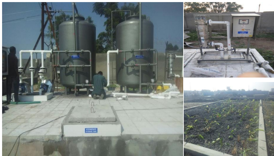
Sara Builders & Developers Pvt. Ltd. - 500 CMD STP
