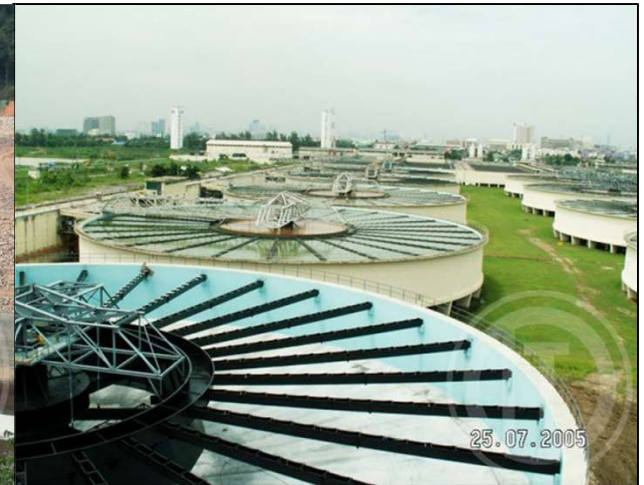
Bang Khen Water Treatment Plant , Bangkok
