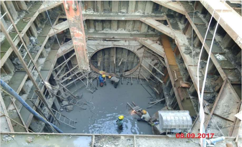
Trunk Sewer KEIP
