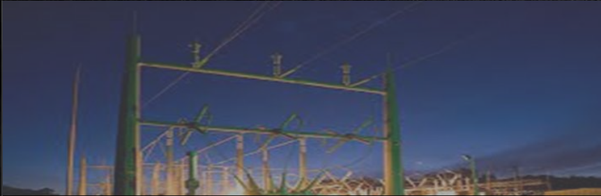
Our E-Houses lighting up a Leading Distribution Company
