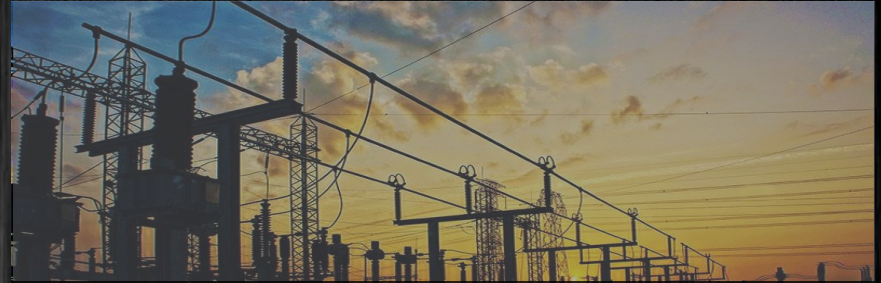
Powering Andhra Pradesh's Future with Substation Supply
